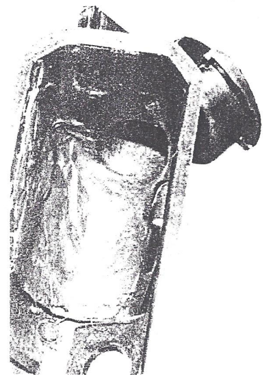
Figure 2 Here we see the inside of a repaired tank, where about 1/4" of Nylobond coating provides much of the strength.
